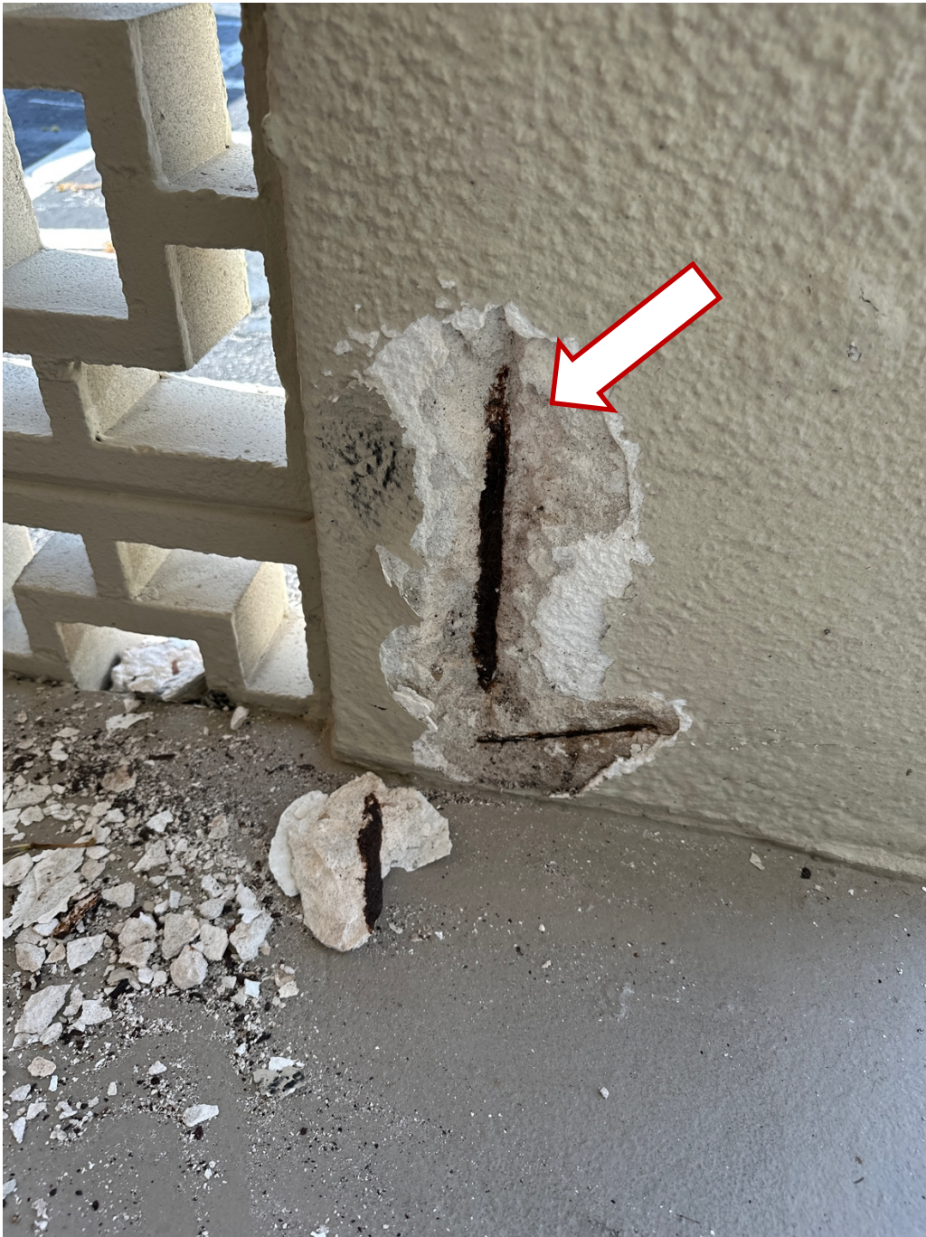
Concrete spall observed at base of column supporting stair landing, ground floor front (South) Capri Isle
