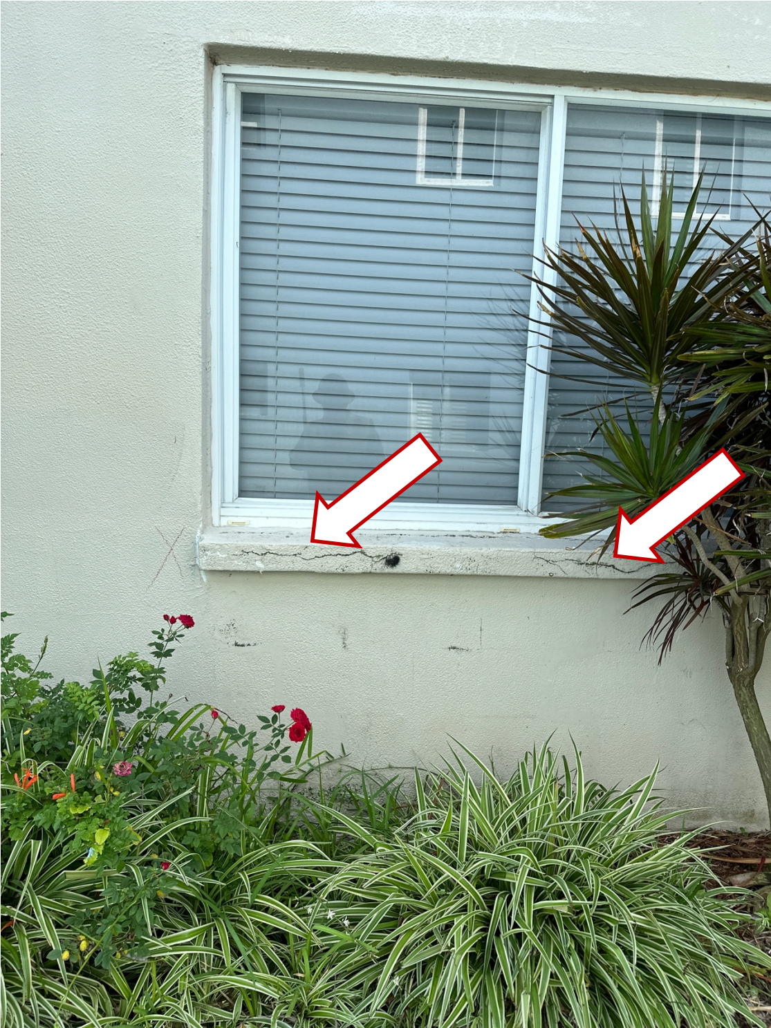
Typical concrete spall in window sill requiring repair (numerous locations on building)
