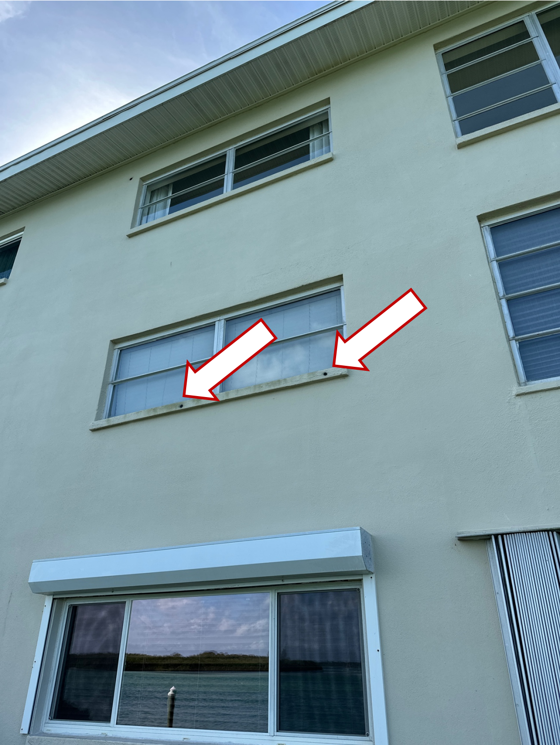
North elevation, Typical concrete spall in window sill requiring repair (numerous locations on building)
