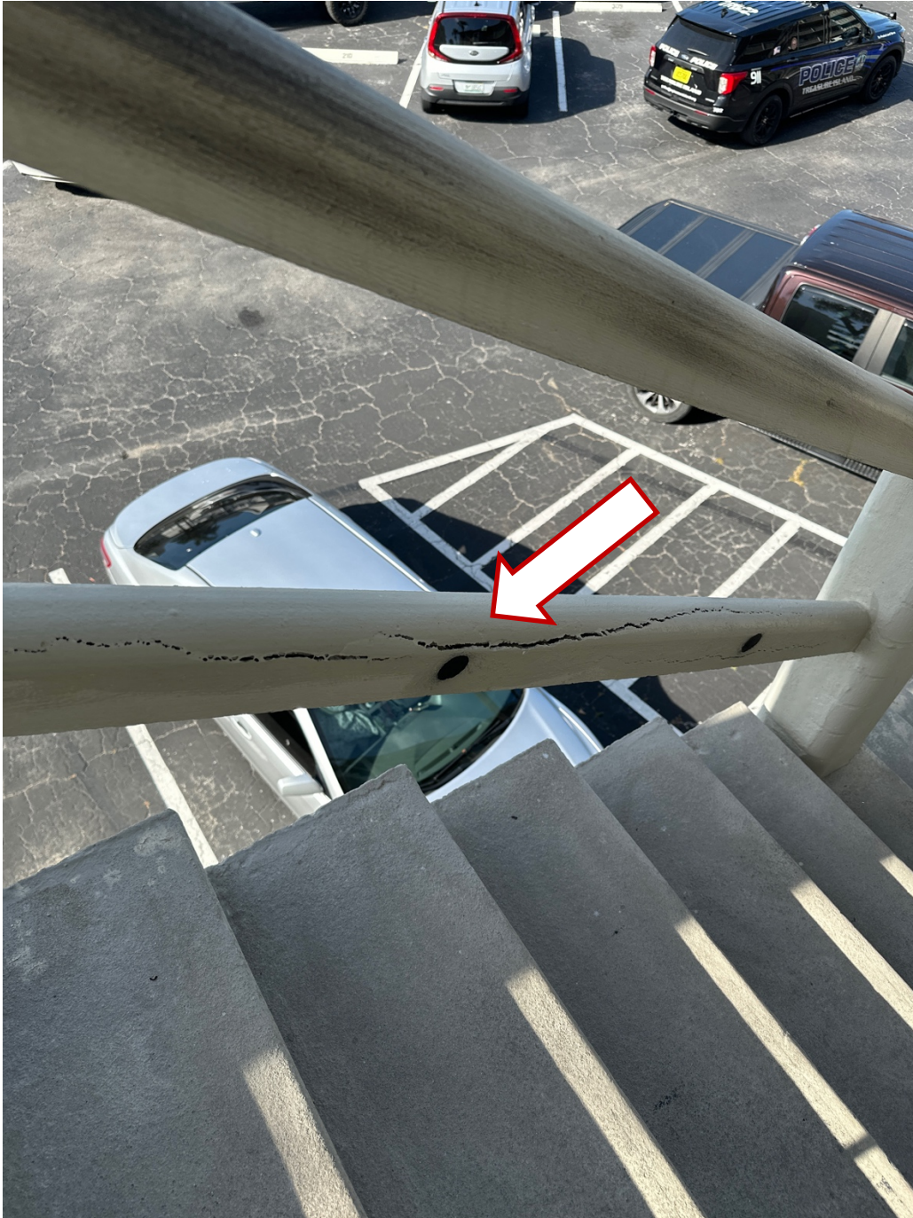
Deteriorated concrete handrail, front (South) elevation, East side. We request direction from Fire Marshal as to whether or not portion can be replaced, or if complete replacement of railing with code-compliant rail is required.
