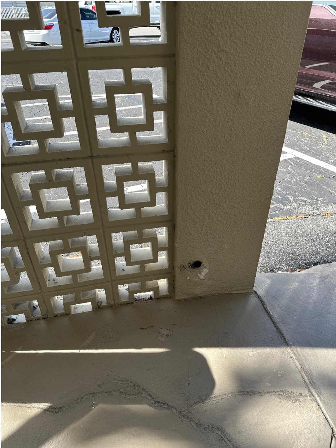
Concrete spall observed at base of column supporting stair landing, ground floor front (South) Capri Isle
