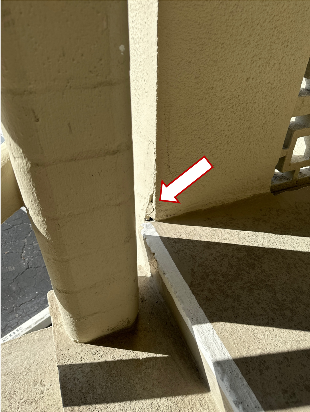
Concrete spall observed at base of column supporting stair landing, elevated stair landing at front Capri Isle
