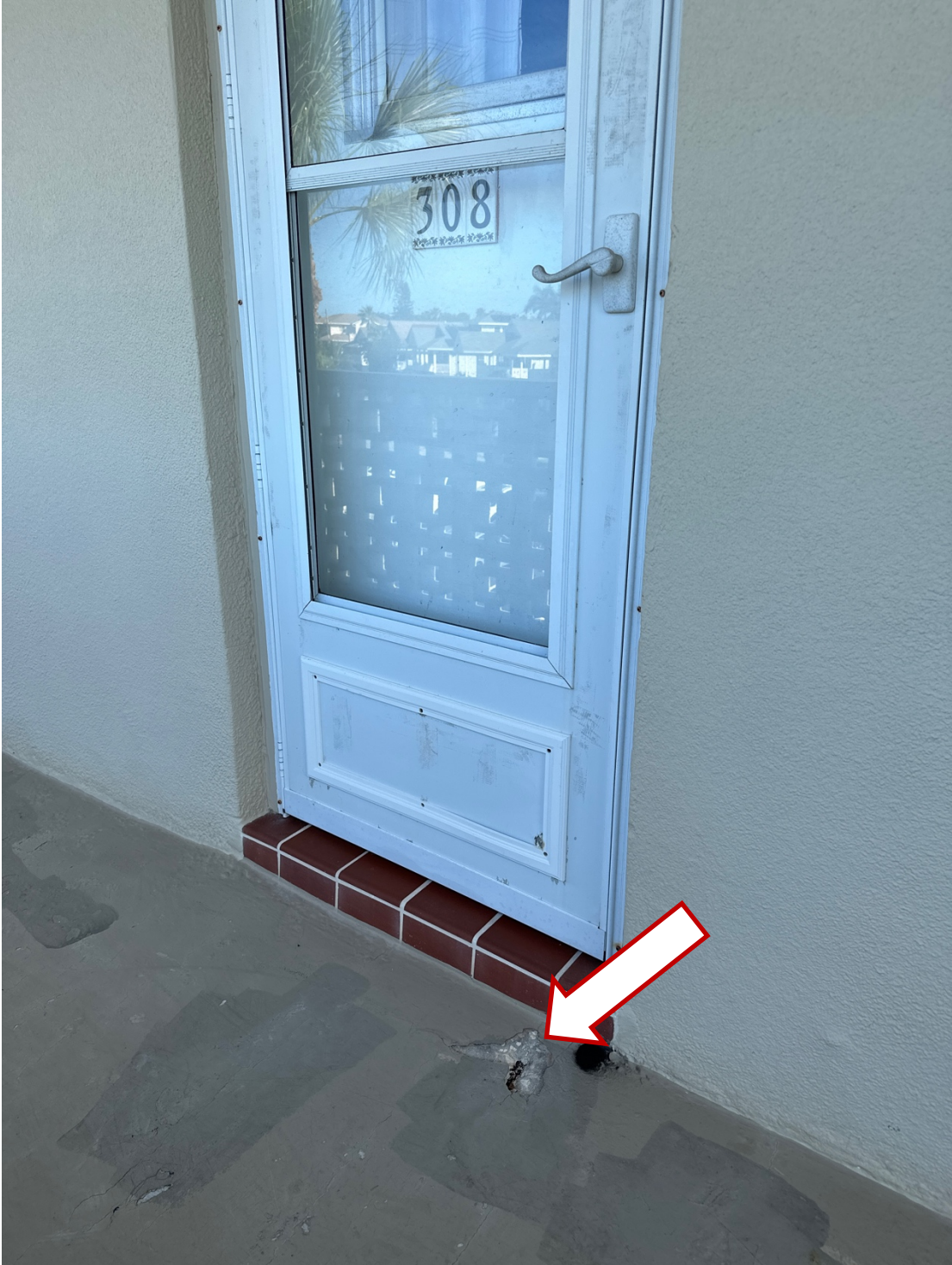
Walkway Slab Repair Location (typical). These will be numerous and their exact locations can only be determined once the walkways are pressure-cleaned.
