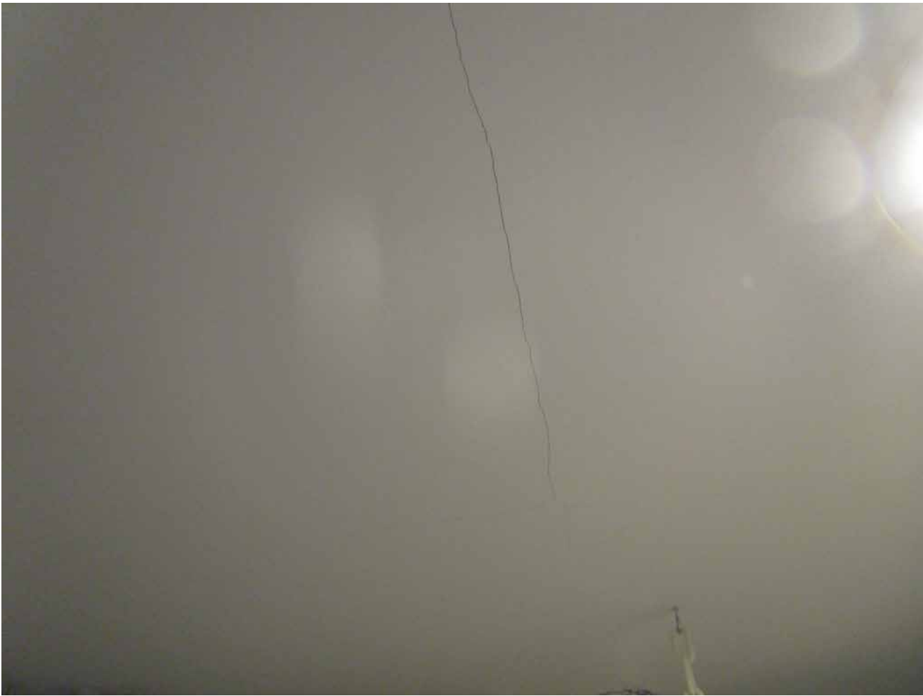
Capri Isle Garden Apartments No. 2. Unit 401. Minor cracking in ceiling observed--not a structural issue and no action is required.
