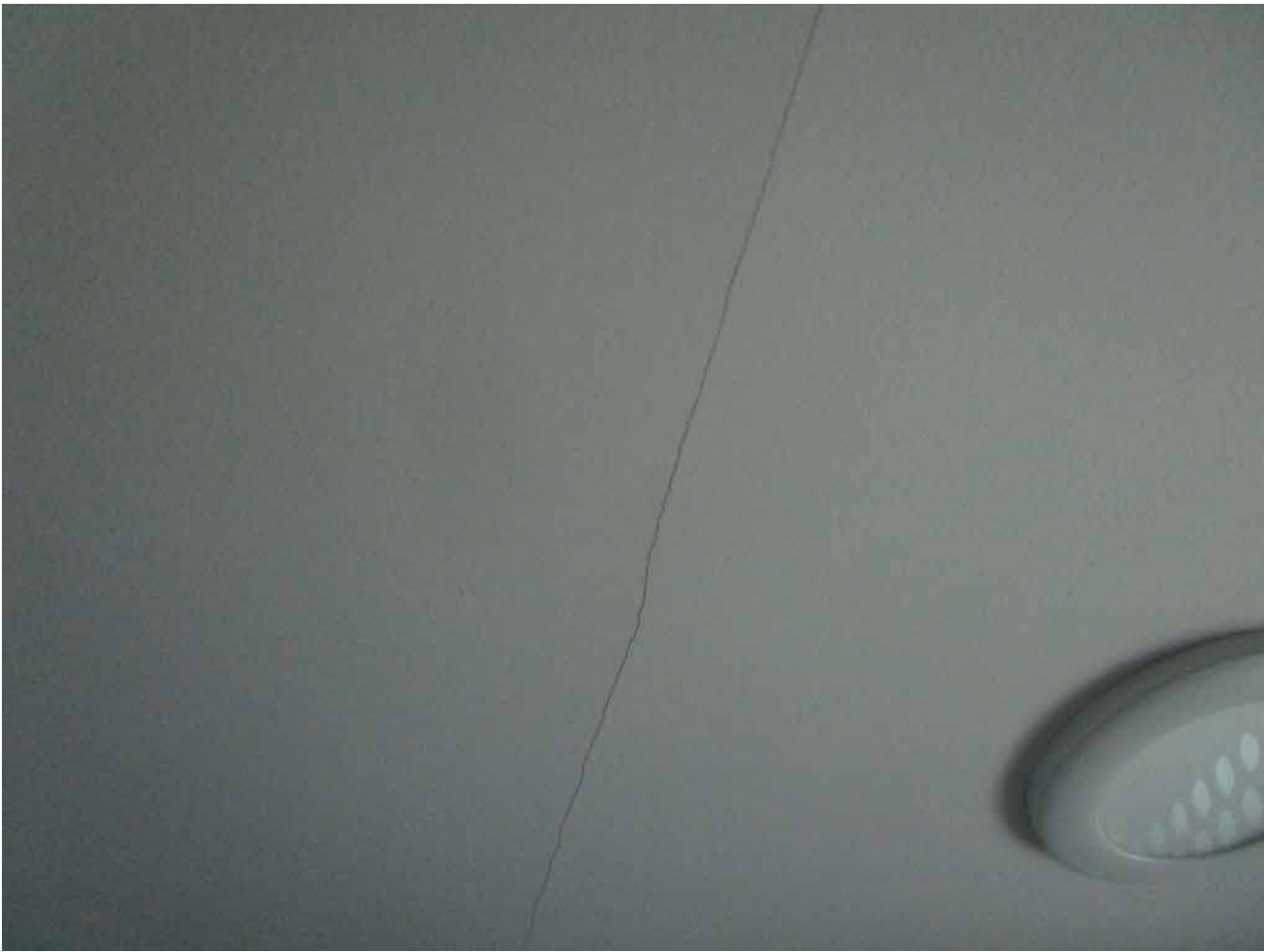
Capri Isle Garden Apartments No. 2. Unit 401. Minor cracking in interior ceilings observed, which is typical for this construction. This is not a structural issue and no action is required.
