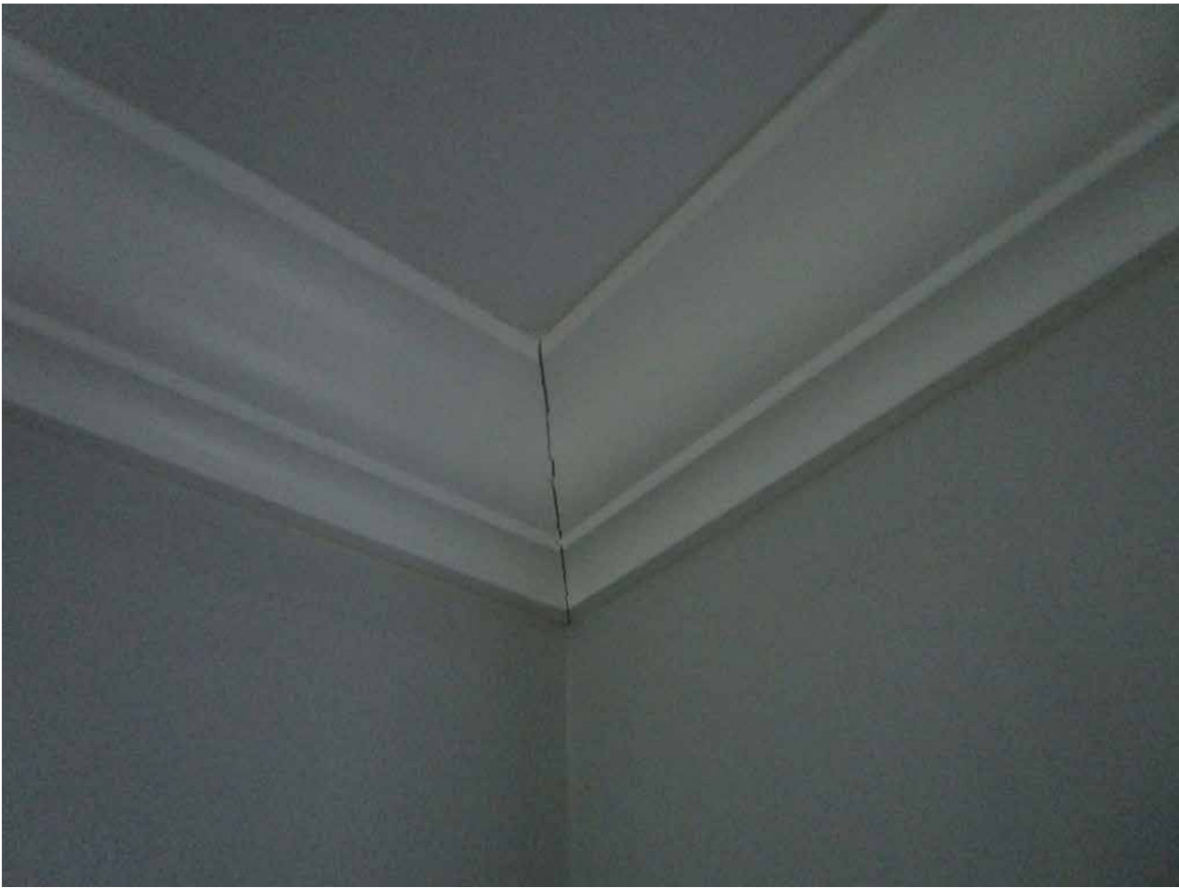
Capri Isle Garden Apartments No. 2, Unit 401. Minor cracking in crown moulding at ceiling. This is a joint where two pieces are joined together. Not a structural issue--no action required.
