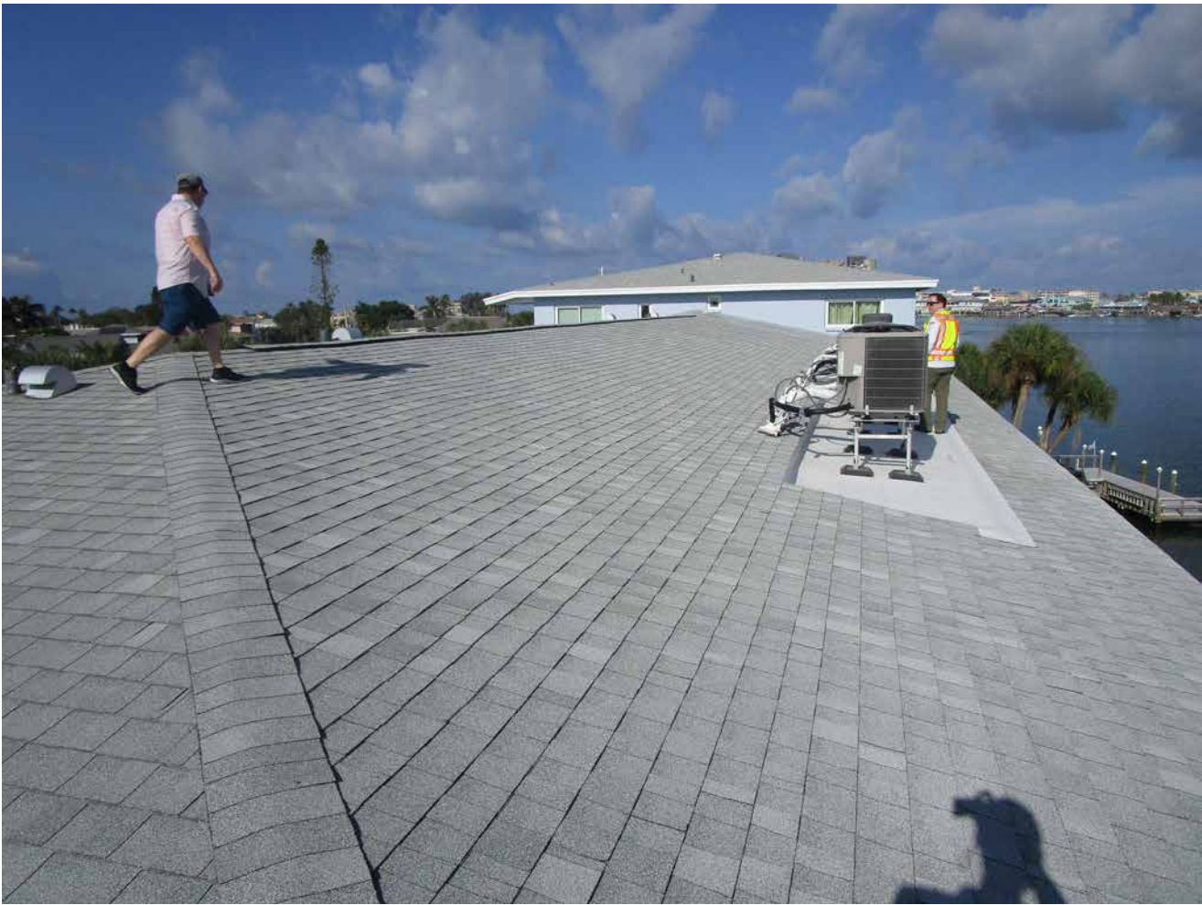
Capri Isle Garden Apartments No. 2. Roof is in good condition. No significant issues observed.
