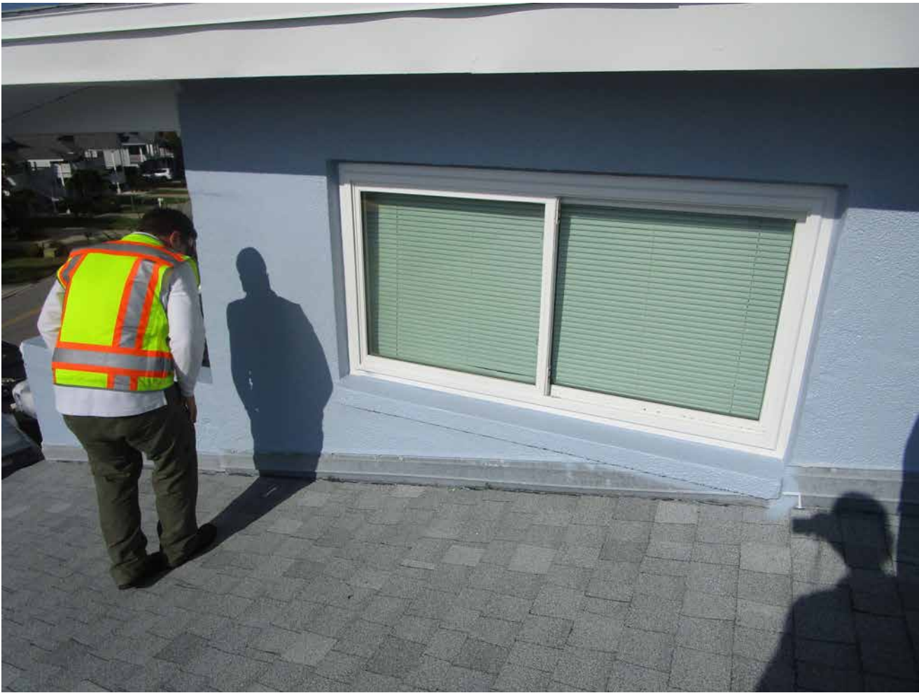
Capri Isle Garden Apartments No. 2. Window perimeter sealants at roof level are deteriorating and reaching the end of their useful life. Recommend removal and replacement of these sealants.
