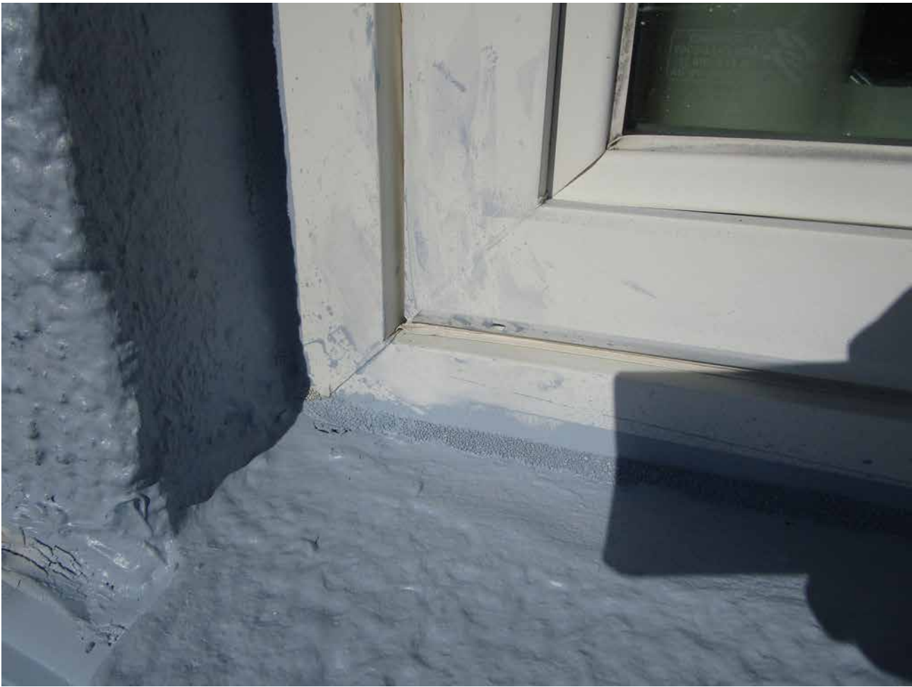
Capri Isle Garden Apartments No. 2. Window perimeter sealants at roof level are deteriorating and reaching the end of their useful life. Recommend removal and replacement of these sealants.
