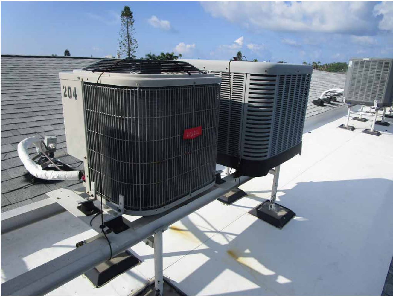
Capri Isle Garden Apartments No. 2. Condensing units are properly secured to roof equipment racks.
