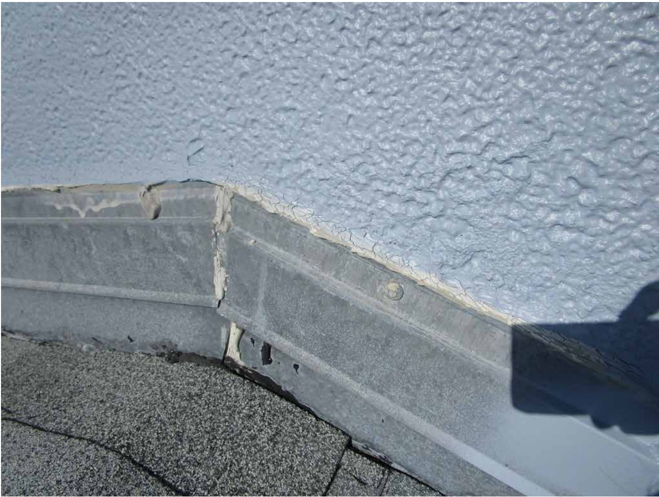
Capri Isle Garden Apartments No. 2. Sealants at top of counterflashing on roof level are deteriorating and reaching the end of their useful life. Recommend removal and replacement of these sealants.
