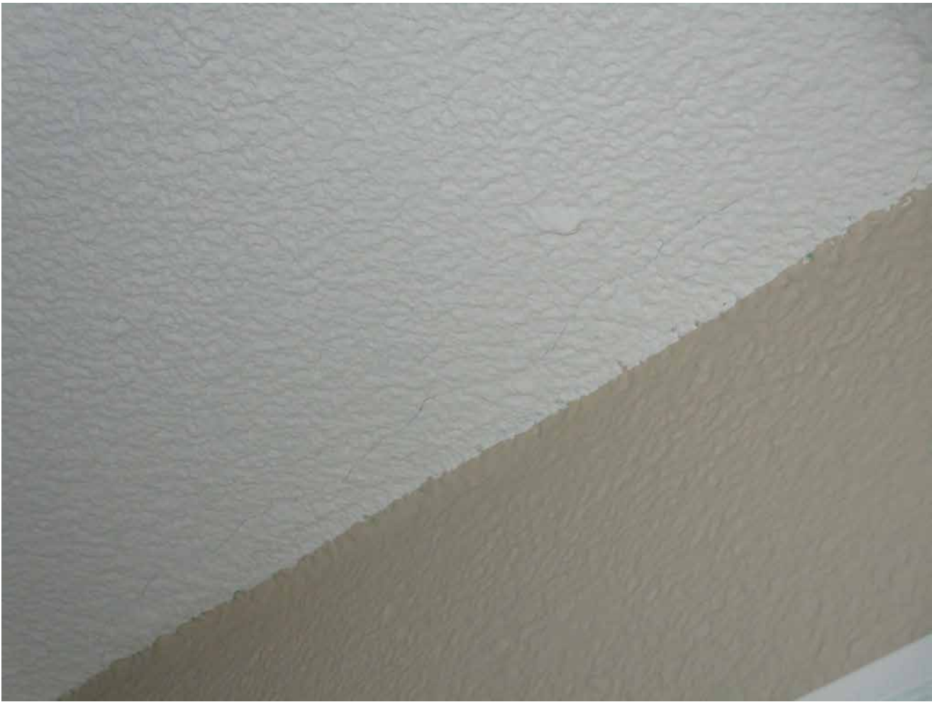
Capri Isle Garden Apartments No. 2. Unit 105. Minor cracking in interior ceilings observed, which is typical for this construction. This is not a structural issue and no action is required.
