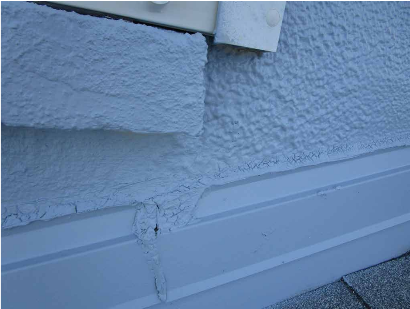
Capri Isle Garden Apartments No. 2. Typical deteriorated sealants at rooftop counter flashing. Recommend replacement as preventative maintenance.
