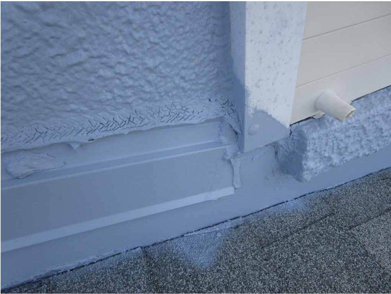
Capri Isle Garden Apartments No. 2. Typical deteriorated sealants at rooftop counter flashing. Recommend replacement as preventative maintenance.
