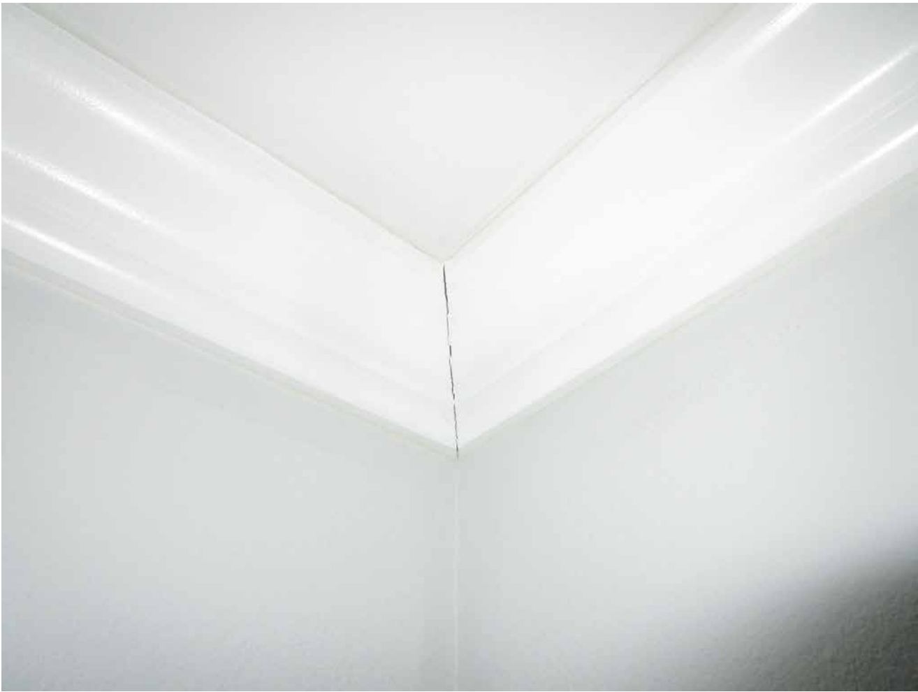
Capri Isle Garden Apartments No. 2, Unit 401. Minor cracking in crown moulding at ceiling. This is a joint where two pieces are joined together. Not a structural issue--no action required.
