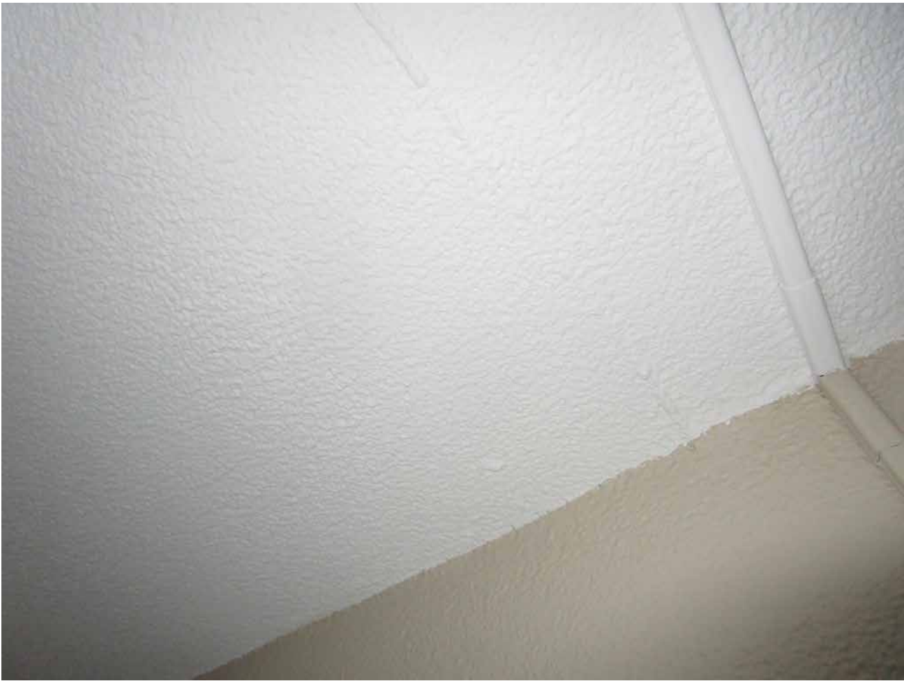
Capri Isle Garden Apartments No. 2. Unit 105. Minor cracking in interior ceilings observed, which is typical for this construction. This is not a structural issue and no action is required.
