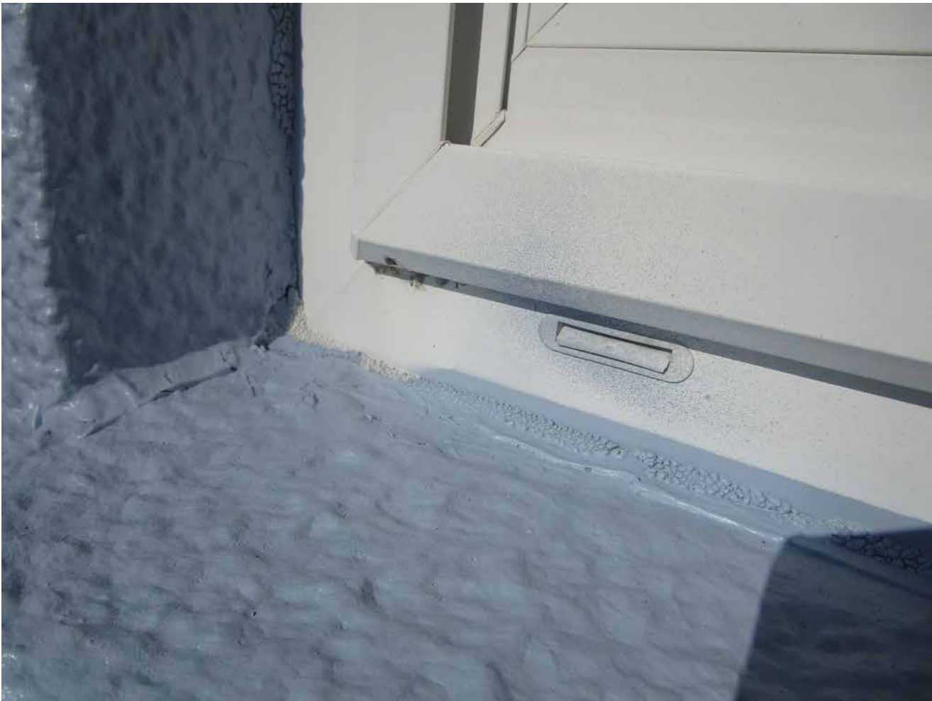
Capri Isle Garden Apartments No. 2. Window perimeter sealants at roof level are deteriorating and reaching the end of their useful life. Recommend removal and replacement of these sealants.
