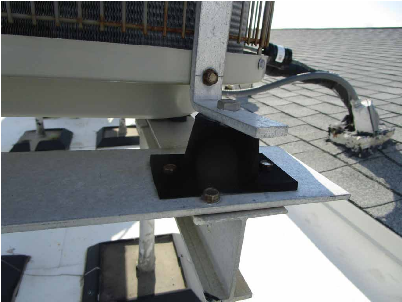
Capri Isle Garden Apartments No. 2. Air conditioner condensing units are properly secured to rooftop equipment rack.
