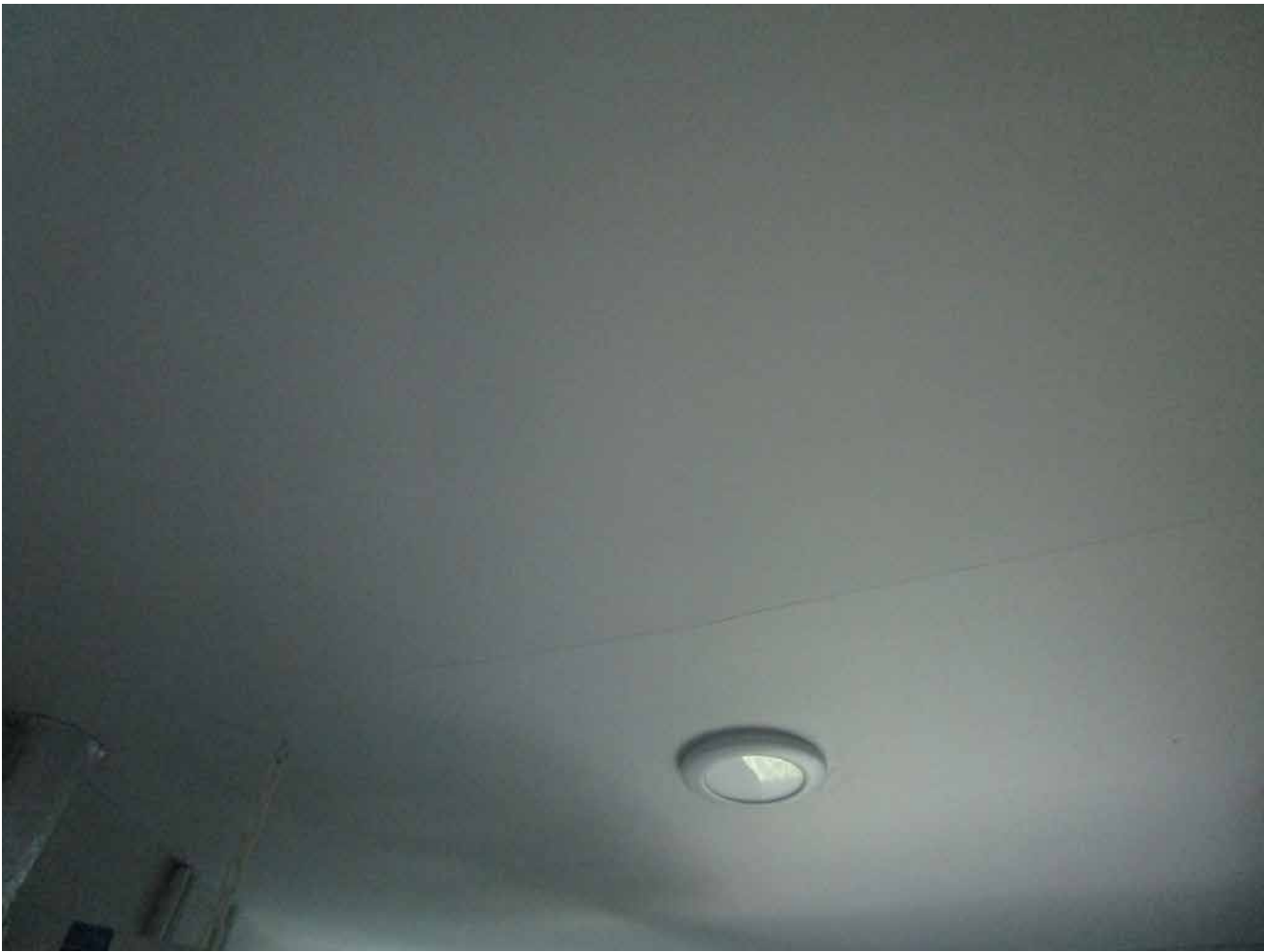
Capri Isle Garden Apartments No. 2. Unit 401. Minor cracking in interior ceilings observed, which is typical for this construction. This is not a structural issue and no action is required.
