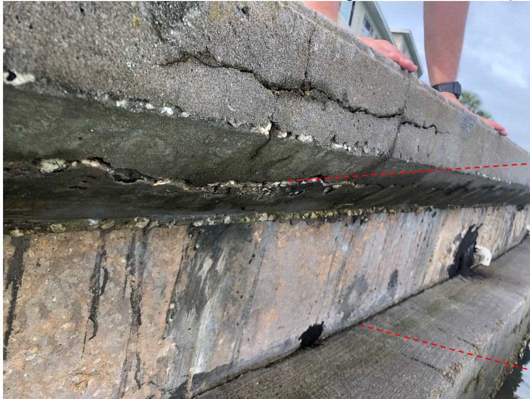
Photo #1- View of the Face and Beveled Edge of the Seawall Cap.
